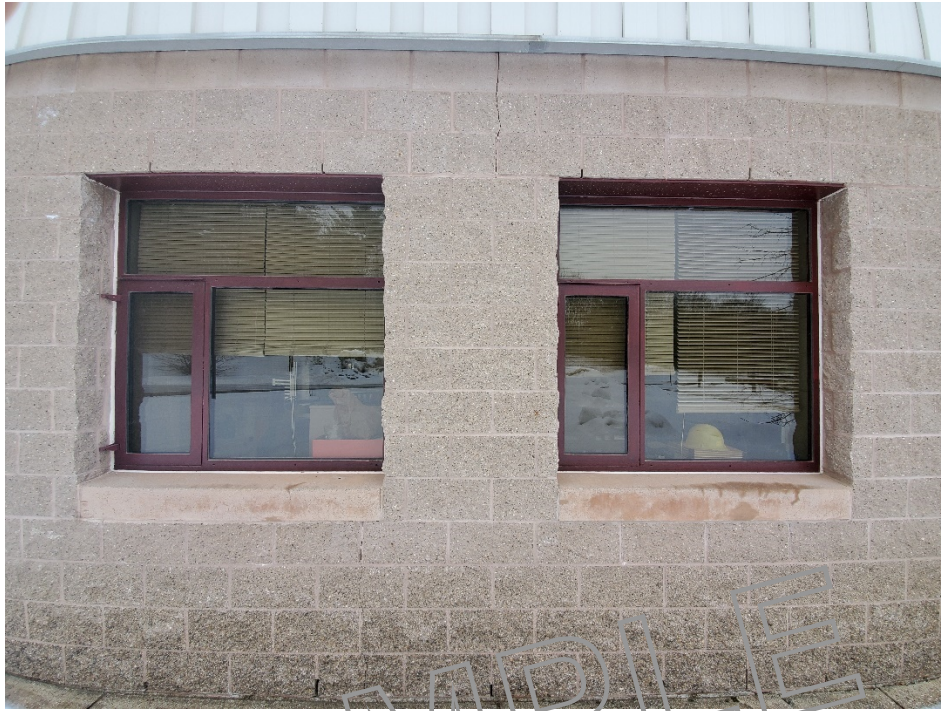
Cracked CMU Above and Below the Windows
