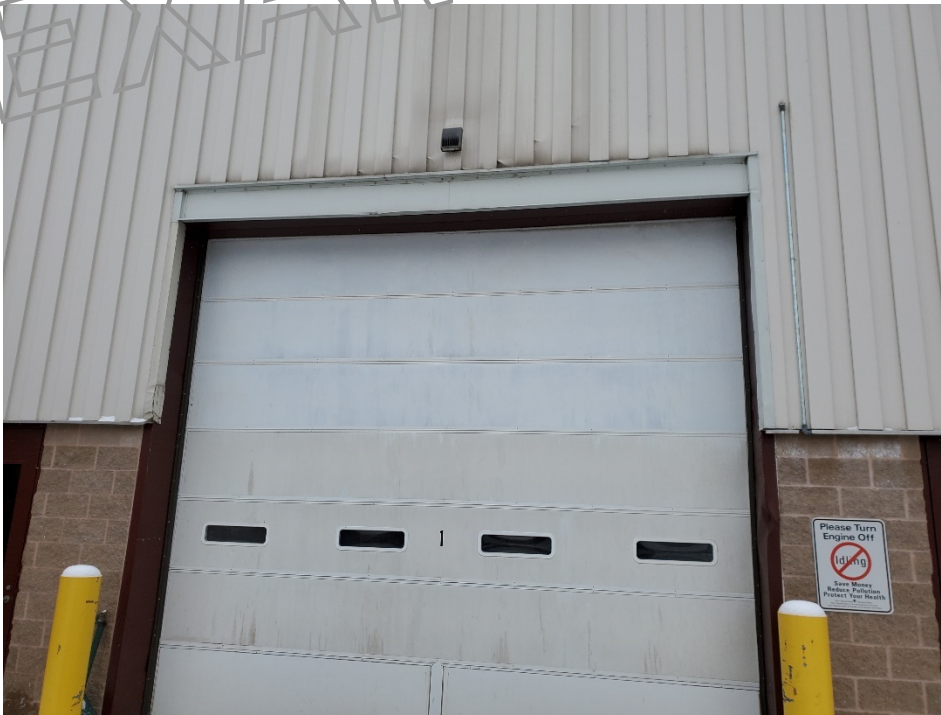
Damaged Siding at Overhead Door
